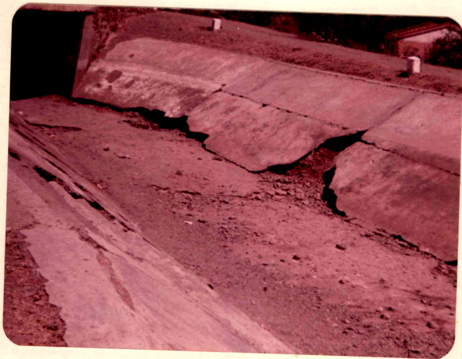
PLATE 1 Cracks in the Right Bank Canal at Wai, near Dhom Colony
