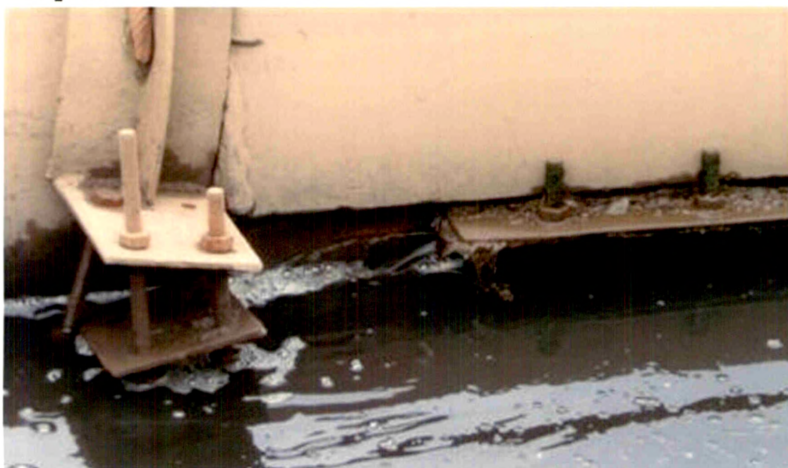
Leakage of effluent carrying pipe line of Lote MIDC.
